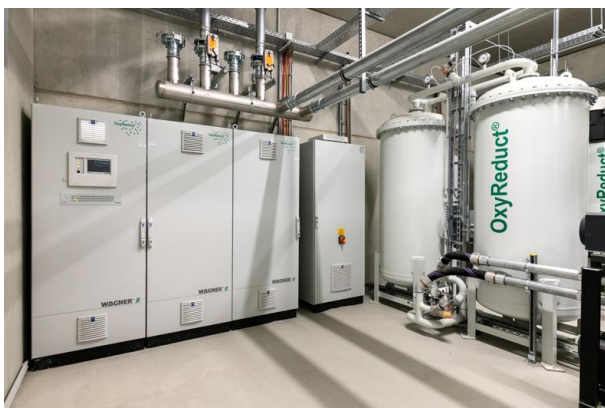
Caption: The OxyReduct® system for active fire prevention in the warehouse requires only a small footprint. Copyright: ©WAGNER Group GmbH
