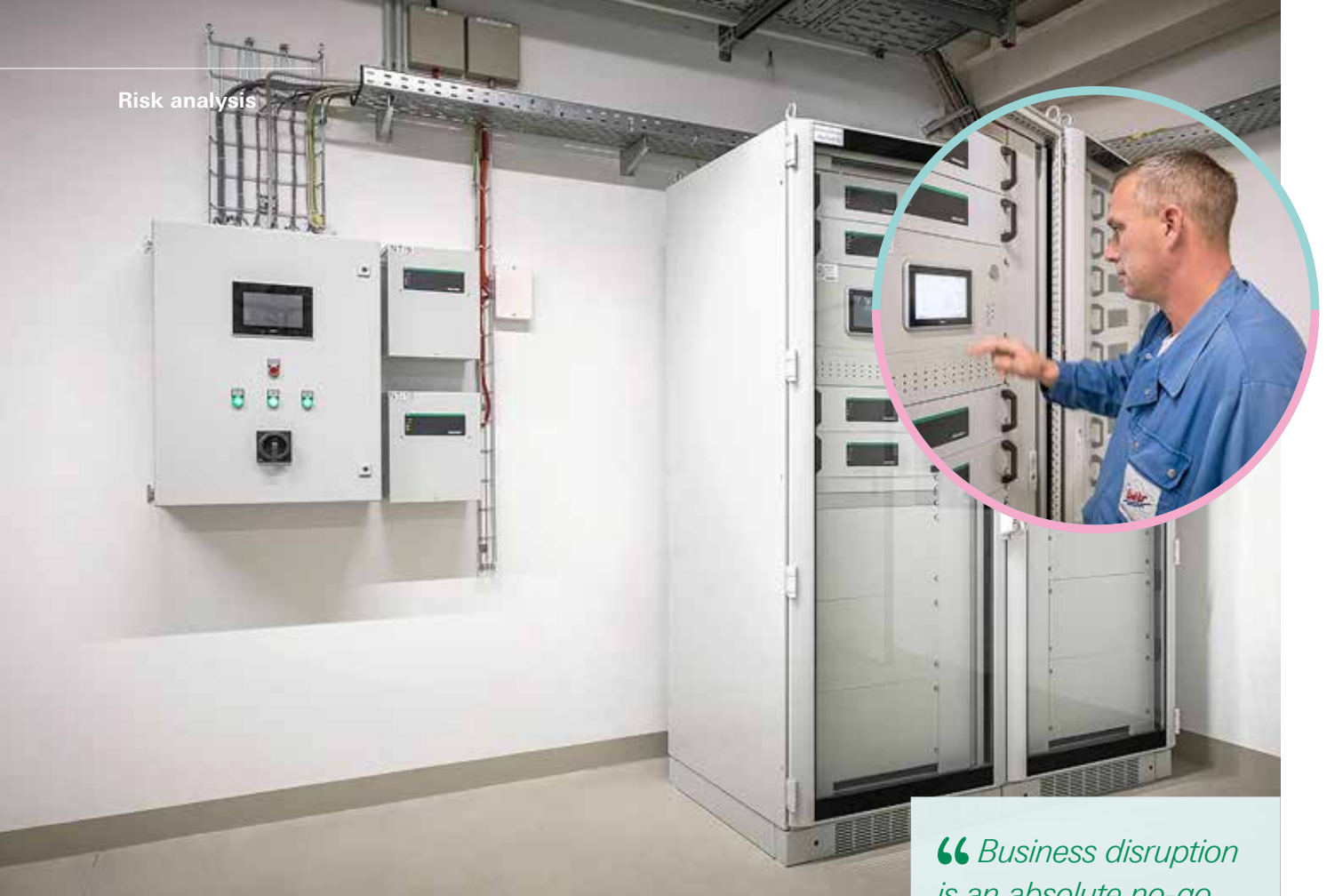
▲ Is really into fire protection: Sebastian Stoll, technical employee of Eisbär Eis, operates the OxyControl centre.
