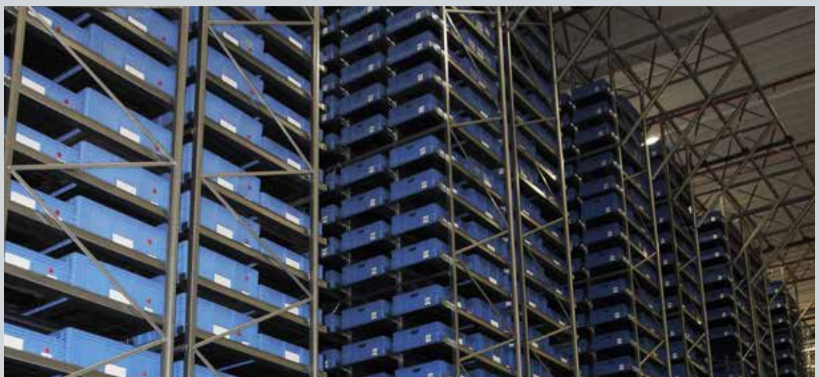
The fully automatic high rack storage with small-load containers is protected from fire danger via an air sampling smoke detector system and active fire prevention.
