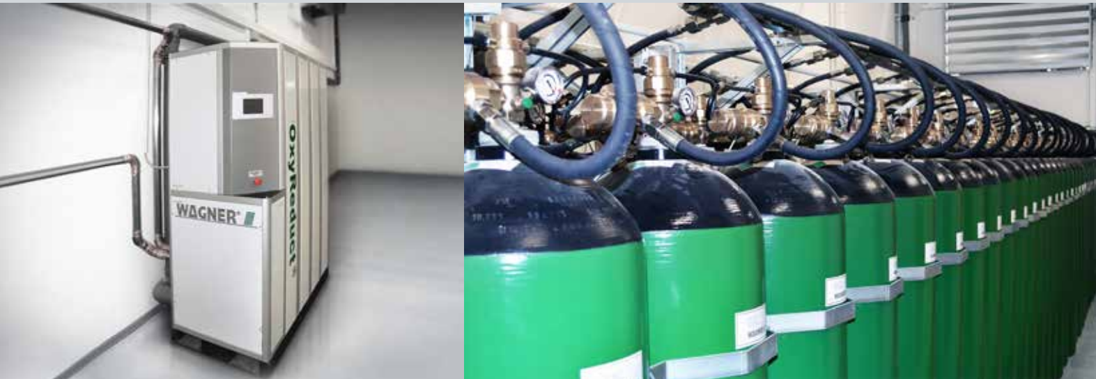
The OxyReduct® active fire prevention system (left) maintains the oxygen content at 16 vol% if a fire is detected. In the event of an additional detection, further nitrogen is introduced to the protected area from cylinders (right) by means of a quick release and the oxygen content is further reduced to 13.5 vol%
