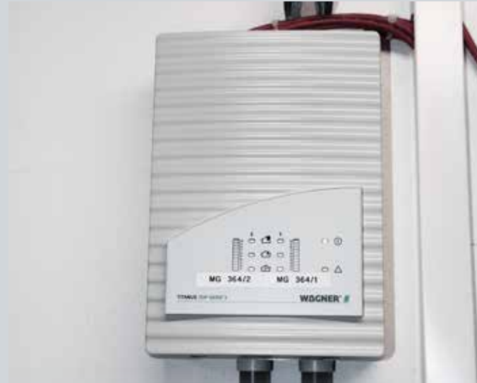
TITANUS® air sampling smoke detectors were installed to monitor the data centre
