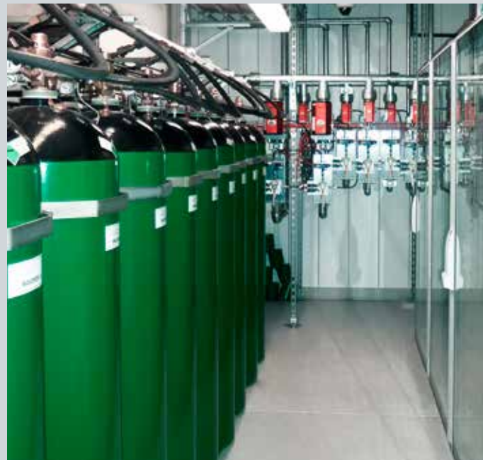
400 kg of nitrogen in cylinders for quick release in ten areas with areas between 10 and 100 m 2
