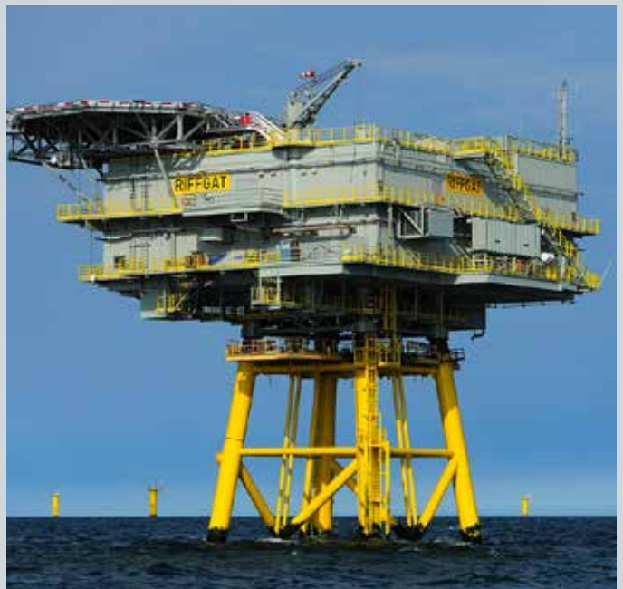
Equipped with fire protection technology WAGNER: The transformer substation at the Riffgat wind farm
